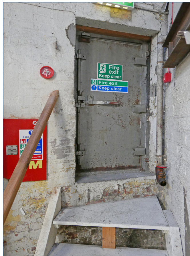
Exit doorway at the south east corner of the Warehouse. This door is immediately north of the Turret.
