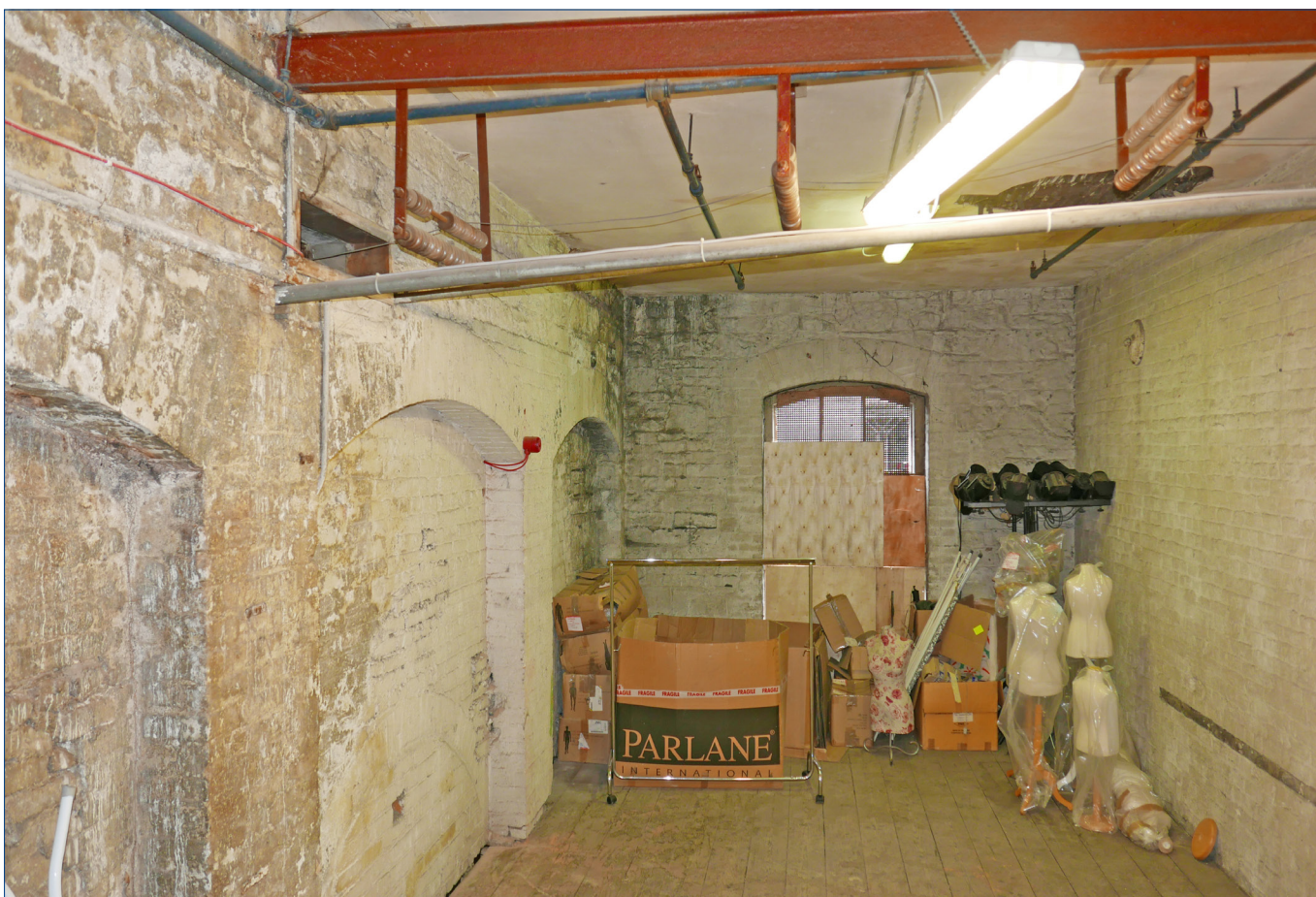
Large gabled building • upper floor • south east corner. The arches to the left are a series in the upper east wall of the large gabled building. The opening to right is in the gable wall facing the river.
