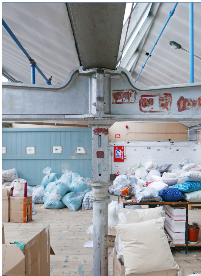
Detail of the joint at the head of one of the Warehouse columns. The ends of two cast iron beams sit on the head of the column and are bolted together. The cast iron gutter runs above, along a valley in the roof.
