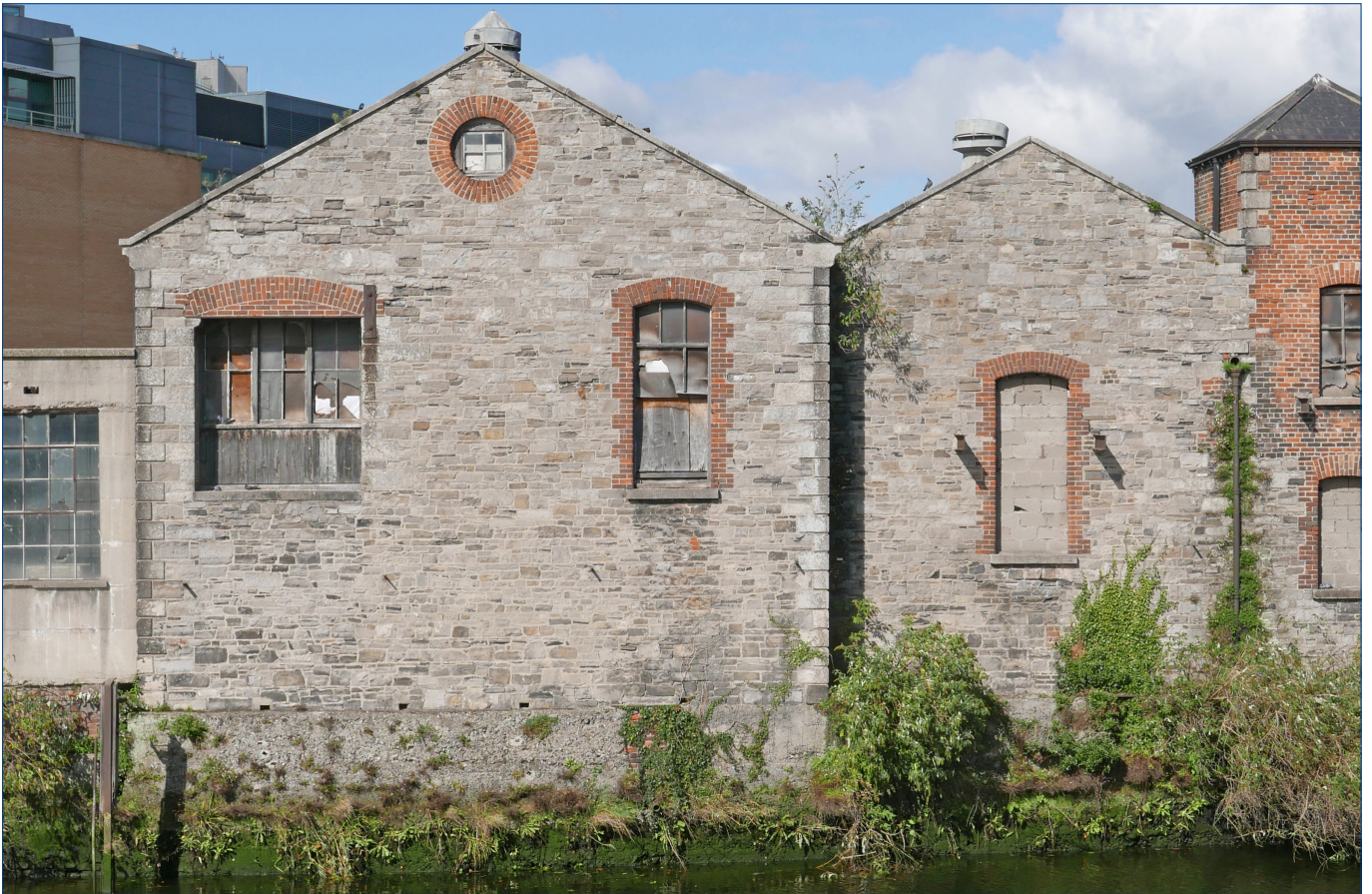
The two Gabled Buildings on the River front first appear on the 1889 Ordnance map and appear to be part of the Kingsbridge Woollen Works, built under the direction of Edward. Cecil Guinness in the mid 1880s. They are built of coursed rubble limestone stonework with granite quoins and sills and brick trim around openings.
