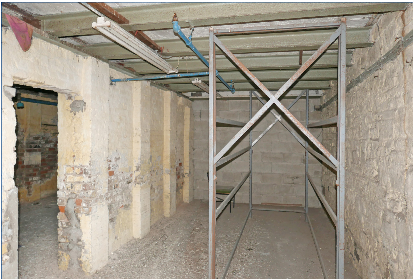
Large gabled building • lower floor • southern 'cellar' on the west side, looking east.
