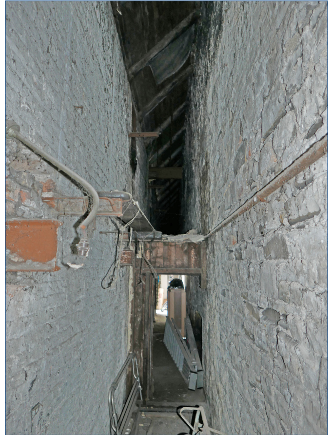
Interior of the space between the Riverside Stone Wall (right) and a separate inner brick wall (left), looking east and upwards near the west end of the Riverside Stone Wall.
