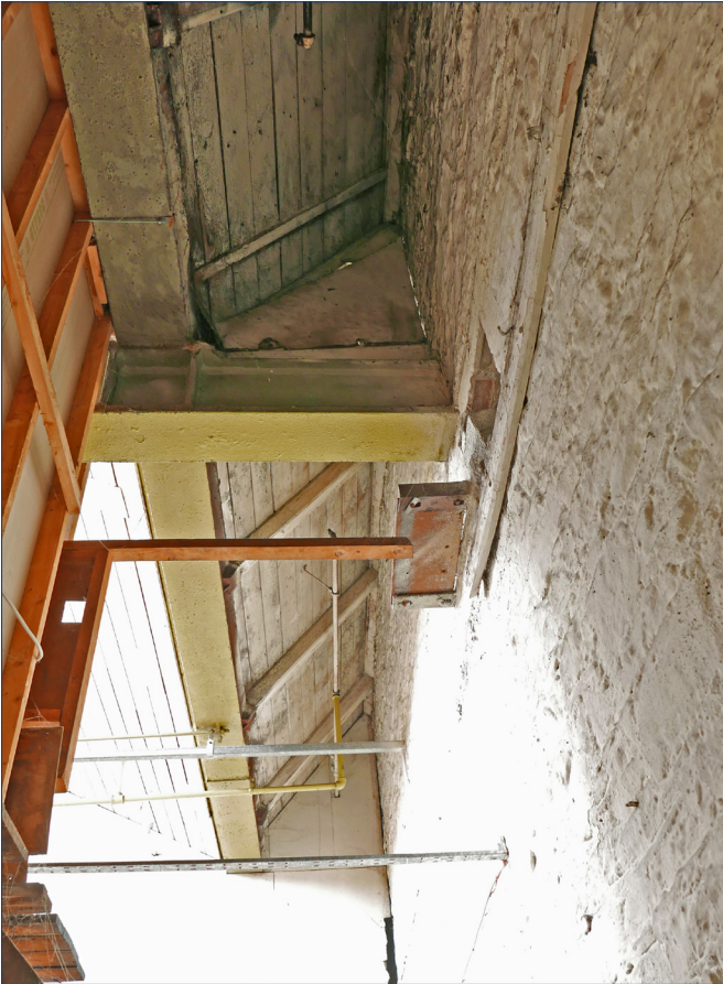
Inside of the Riverside Stone Wall, looking east and upwards near the east end of the wall. At the east end of the warehouse, two cast iron roof beams continue to the Riverside Stone Wall. The rest of the beams do not
