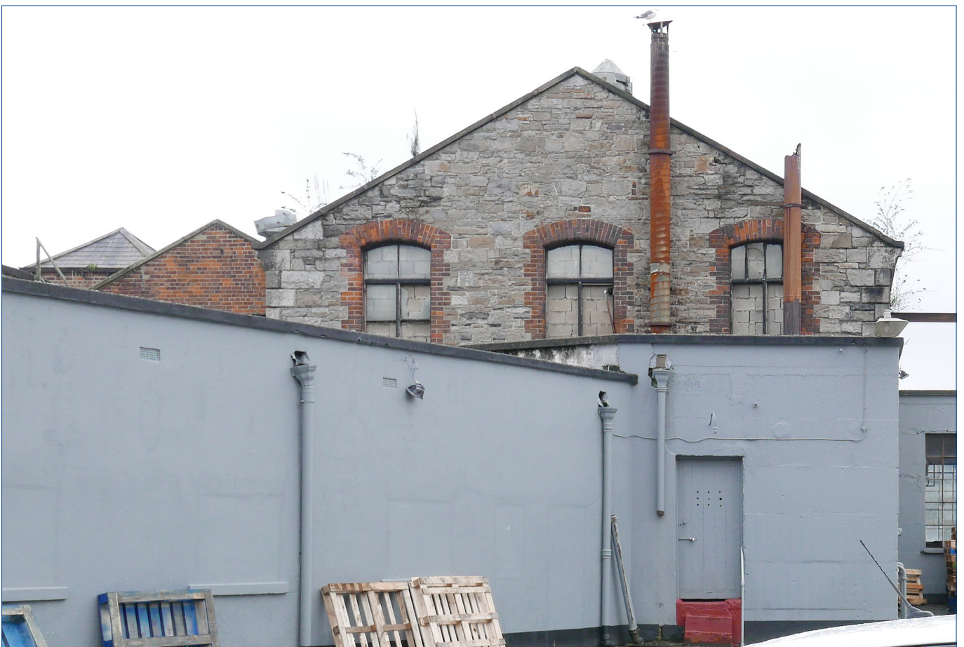
Large gabled building • upper part of the north facade seen over the grey walls of single storey structures in the foreground. The brick gable seen to the left is the north gable of the smaller gabled building. The top of the square tower is seen on the extreme left.
