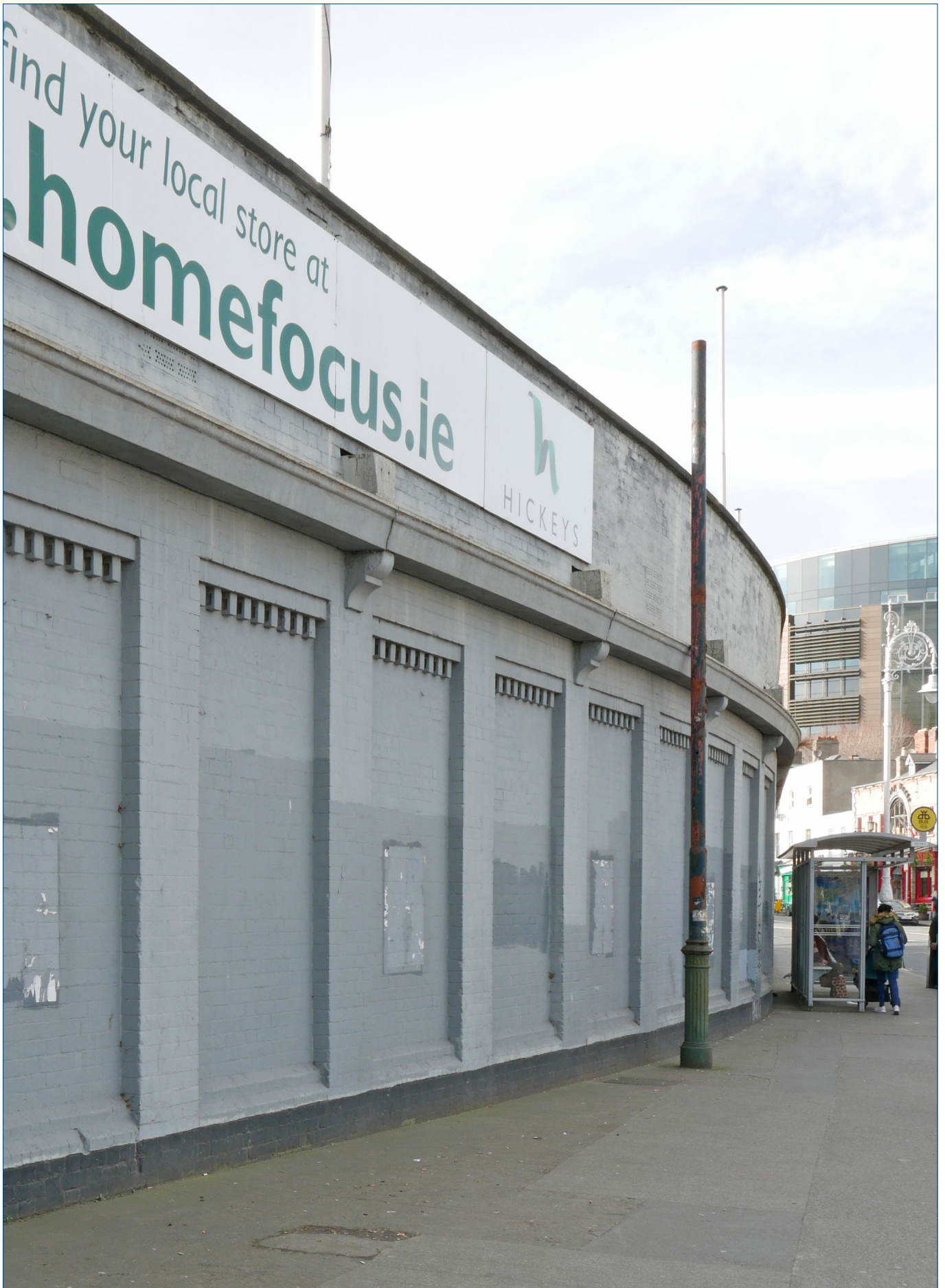
Outer face of the warehouse wall curving along the south side of Parkgate Street. A continuous cast iron gutter is seen supported on carved granite corbels, with the end of one of the cast iron valley gutters of the northlight roof emerging above each corbel. Every second pier in the brick wall supports a corbel, and is aligned with one of the cast iron valley gutters of the northlight roof. As the wall curves along the street, the separation of the brick piers varies, so that every second pier maintains alignment with a cast iron valley gutter.
