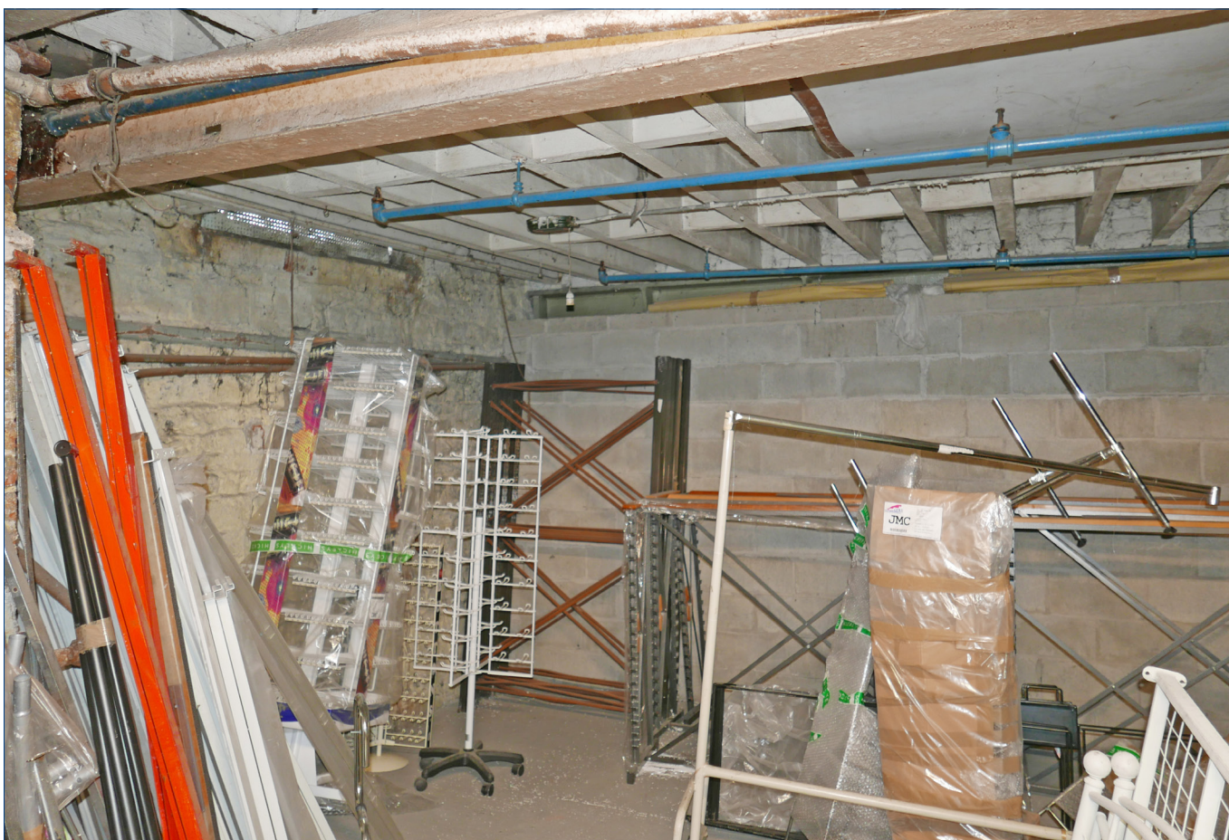
Large gabled building • lower floor • space at the south east corner, looking south west.
