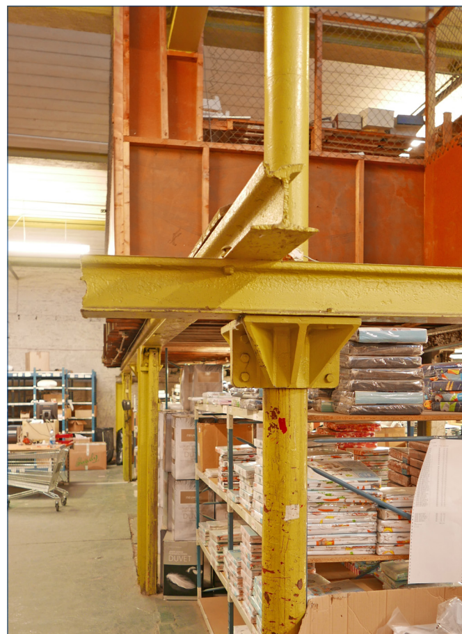
Mezzanine structure near the south west corner of the Warehouse. One of the main columns is seen with a collar supporting two lengths of tram track passing at right angles.
