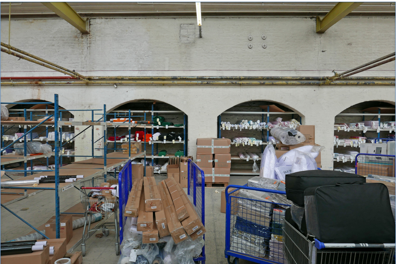
View in the Warehouse, looking south towards the arches in the separate inner brick wall. In all but two cases, the cast iron beams supporting the roof stop at the inner wall and do not continue to the Riverside Stone Wall.
