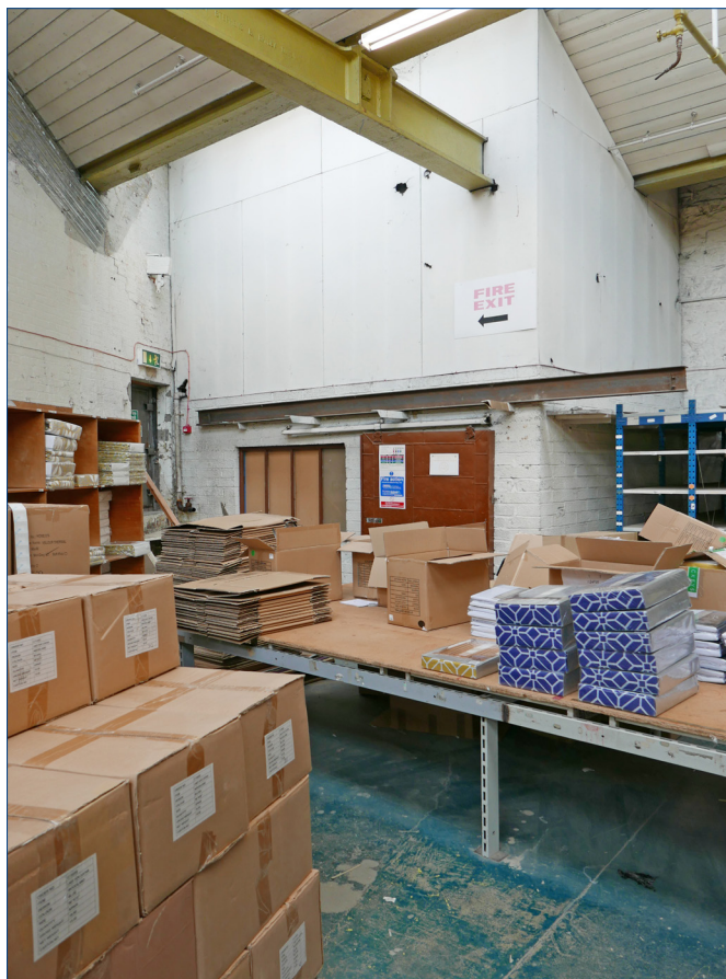
South east corner of the Warehouse. The corner, where the Turret is located, has been walled off in modern blockwork to provide a tank room.
