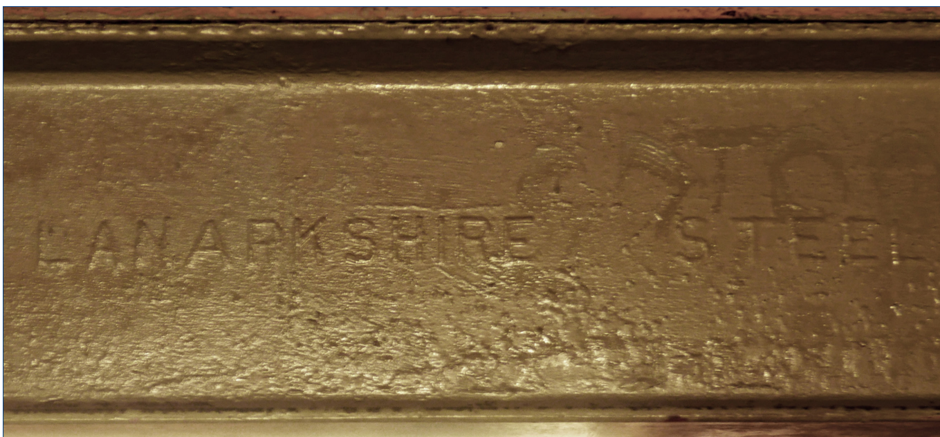
The name 'Lanarkshire Steel' marked on a rolled steel joist near the western side of the Warehouse.
