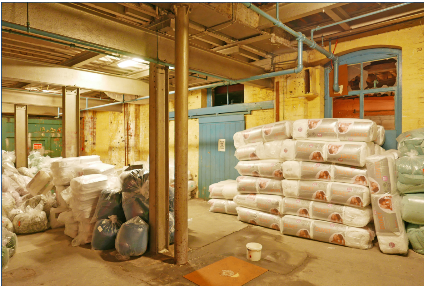
Large gabled building • lower floor • space at the north end, looking north west. The photo shows the north west corner of the building with three openings in the north wall. The round column in the centre of the image carries a beam that supports the north end of the east side of the upper wall of the large gabled building. The blue window to the right is not within the gabled buildings.
