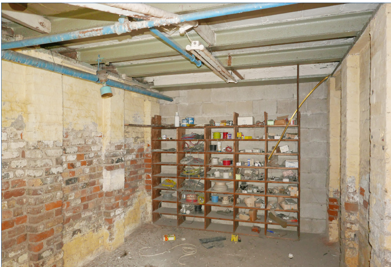
Large gabled building • lower floor • centre 'cellar' on the west side, looking east
