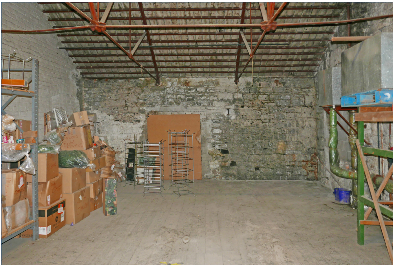
Large gabled building • upper floor • space at the north end of the building, looking west
