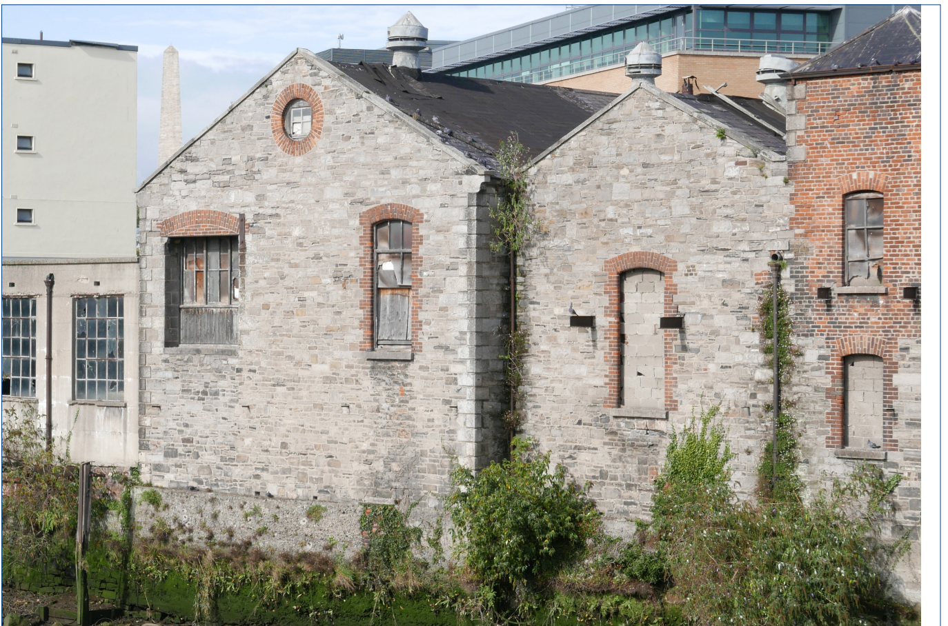
The Gabled Buildings address the River, and there is clear evidence from these photographs that they were used for loading and unloading goods from wharfs that would have run along the river below them. The slate roof of the Square Tower appears largely intact, but it appears that the roofs of the gabled buildings have been felted over, at least in part.
