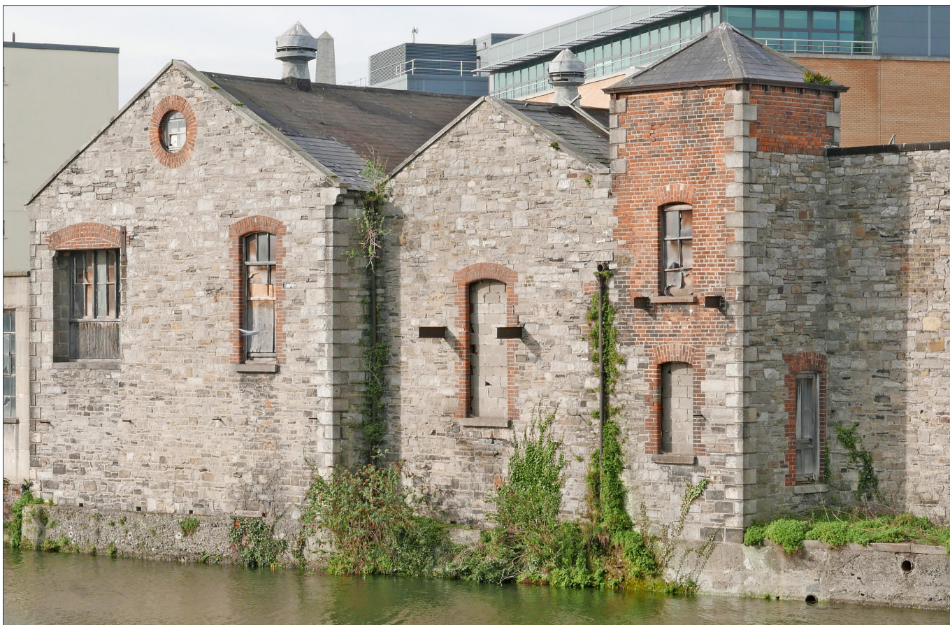
Oblique view of the river buildings, north west. The image shows the opening in the east side of the Square Tower. The shape of the shadow of the square tower on the river wall suggests that the upper half of the river wall tilts back at that point. There is an opening on the east side of the Square Tower, a former door or window. It is proposed to fit a simple modern window into this opening.
