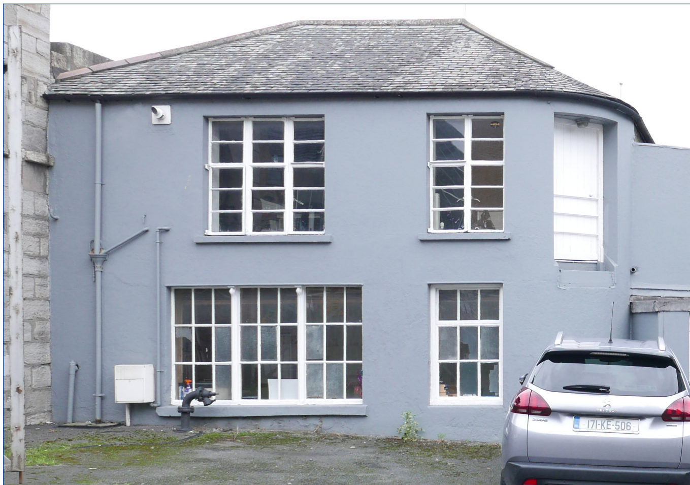
West side of the small two storey building located inside an east of the Stone Arched Entrance Gateway. The windows are of different dates, with the three part lower window to the left being the earliest
