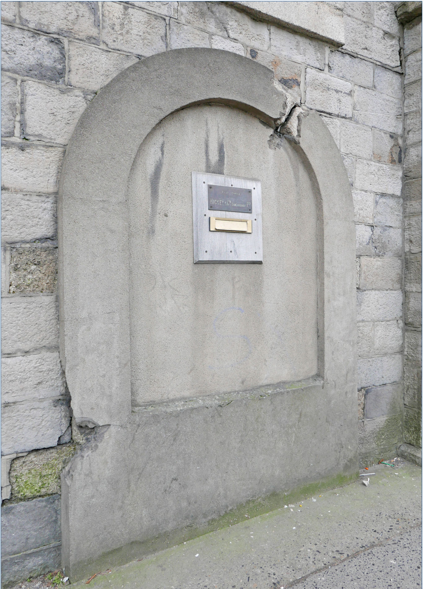
Rendered area covering part of the eastern flank wall to the Stone Arched gateway. Perished granite stonework can be seen where areas of render have come off. The render may be concealing a round headed doorway, a window opening, or possibly a recessed panel.
