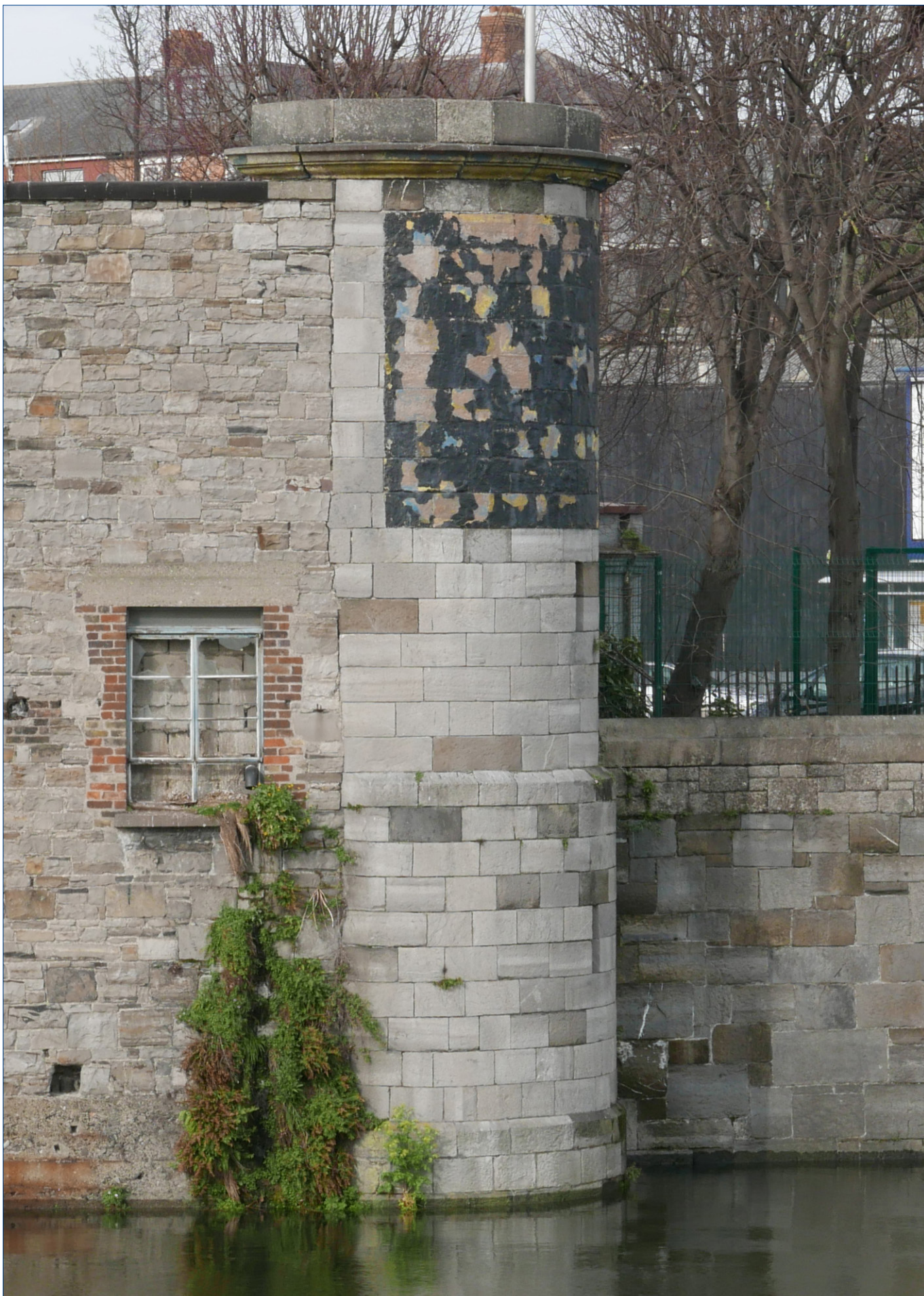
The turret is constructed in the main of cut limestone in an ashlar pattern. The cornice and blocking course are in granite. The Turret appears visually to be in relatively good condition though there is a need for some careful non-aggressive stone cleaning, removal of plants, and minor stone and pointing repair.
