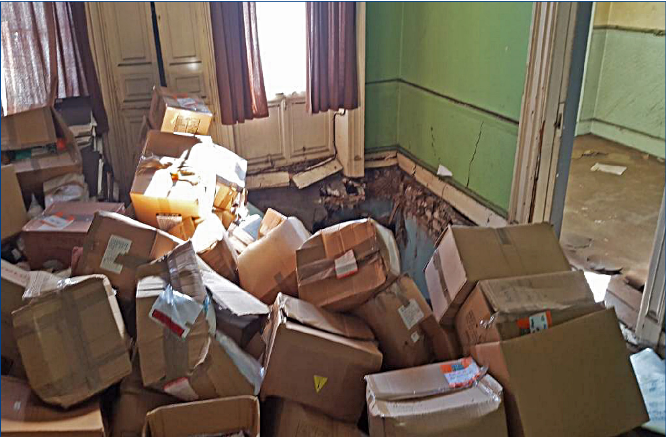
Interior view of 'Kingsbridge House' showing the ground floor partially collapsed into the basement. This image is from a report dated September 2016 by DBFL Consulting Engineers.
