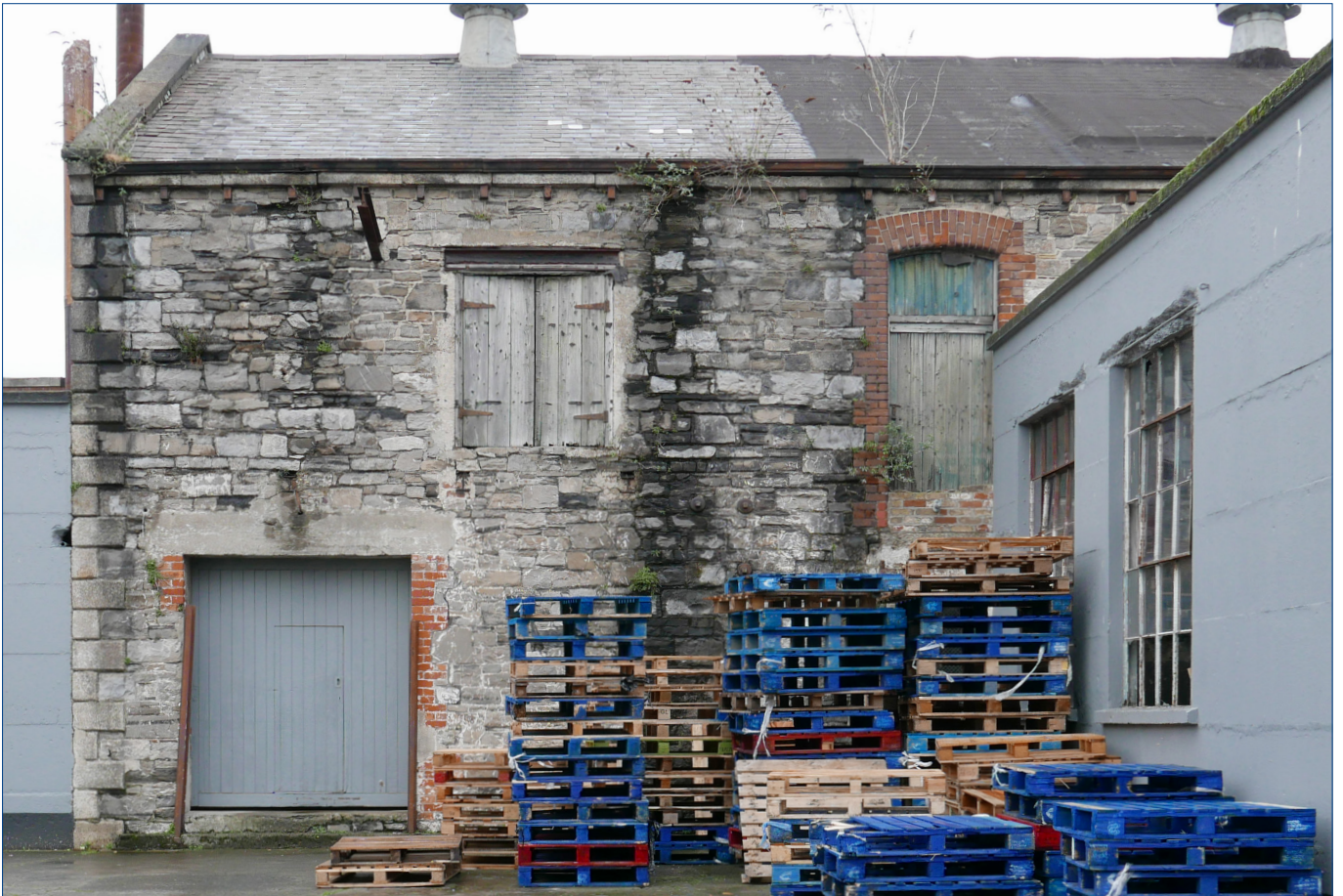
Large gabled building • north end of the west facade. Of the three openings seen in this view, only the opening to the right, with the brick trim, appears original..The stonework is in need of cleaning, repair and repair of pointing. The slated roof needs to be repaired and reinstated.
