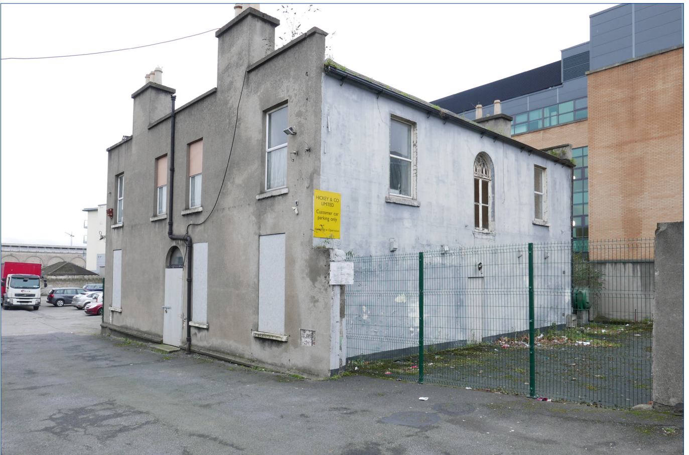
'Kingsbridge House' as seen from the north east. Ordnance mappings shows buildings, now gone, covering the yard to the right, between the house and Parkgate Street. The house is in very poor condition and is structurally failing internally.
