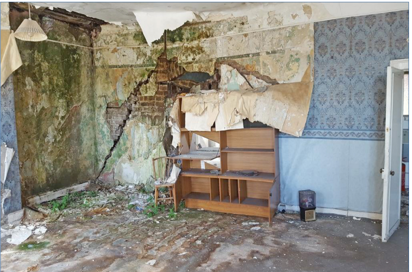
Interior view of 'Kingsbridge House' showing the structural failure of an internal spine wall. This image is from a report dated September 2016 by DBFL Consulting Engineers.
